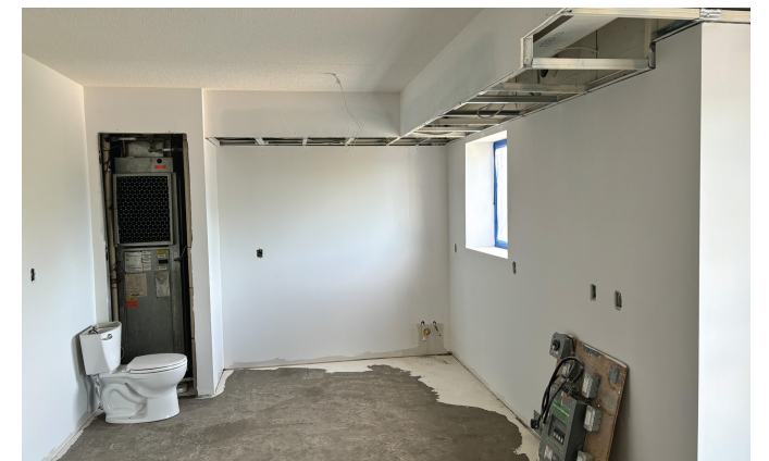
Through generous support from our community, SHOW has begun the rebuilding process and is looking forward to welcoming a new resident home in 2025
