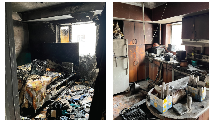
A devastating fire completely destroyed a unit at 362 Erb St. W.
